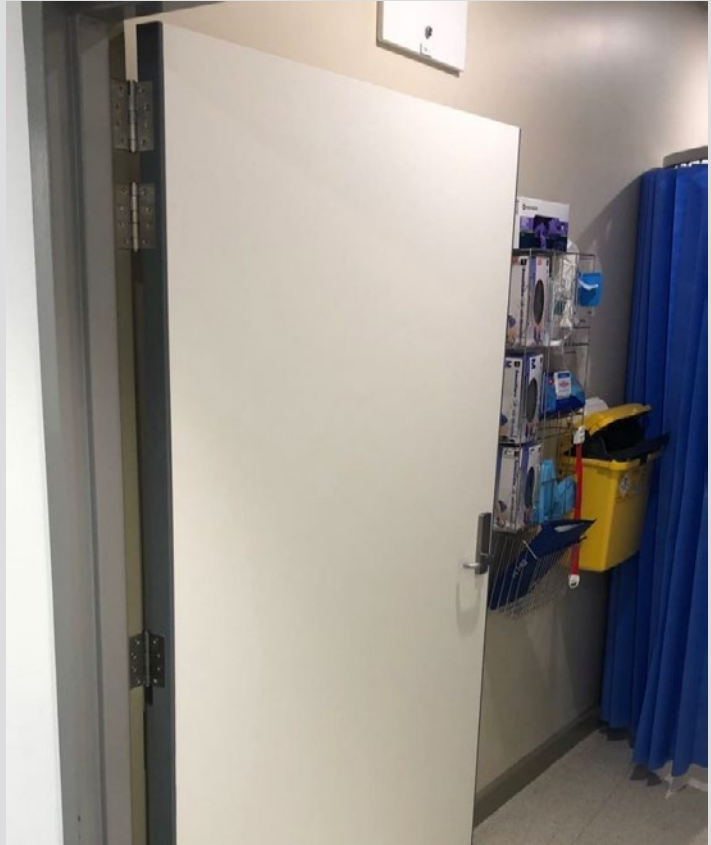
New "Fully Sealed" doors fit perfectly into openings after being Laser Scanned
